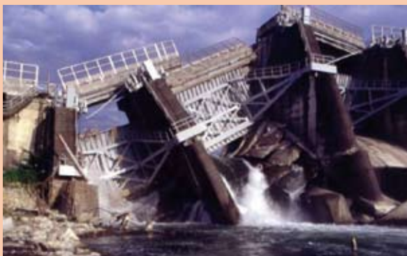
Collapsed dam in a Taiwan Earthquake
